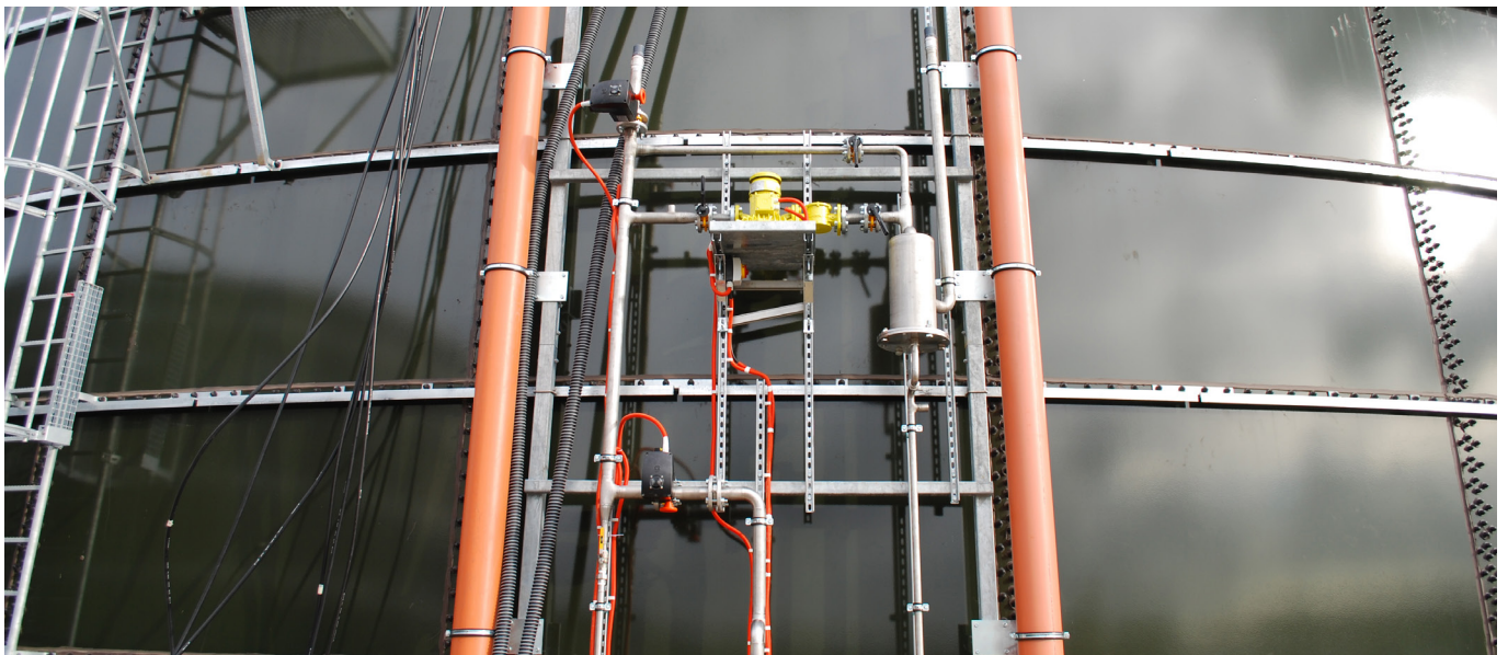
Gas compressor system / Gasverdichtersystem
